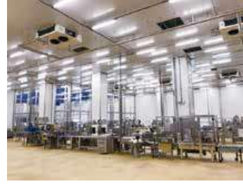
thermofin air coolers with double coil
